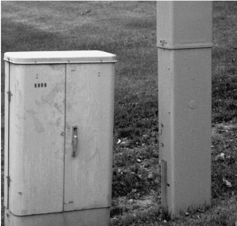
Figure R.10 Repeater Closure (Left) and Splice Pedestal (Right)
