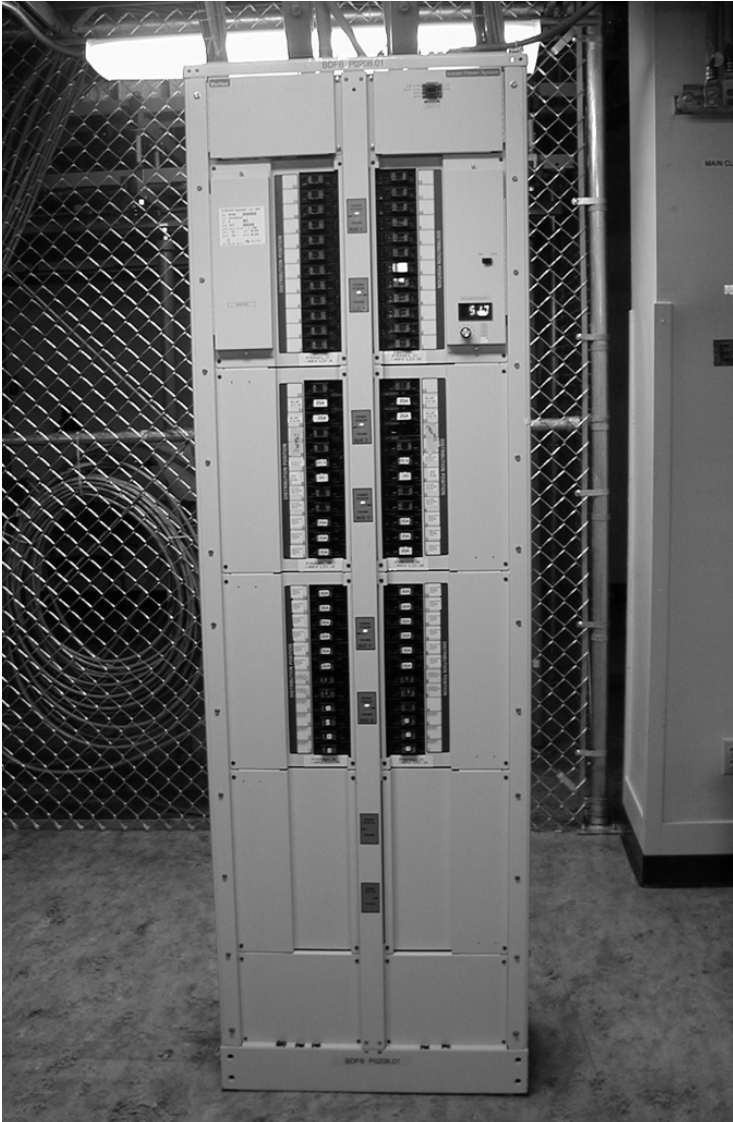
Figure B.11 Breaker Distribution Fuse Bay (BDFB)
