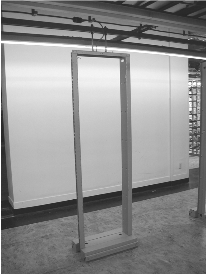
Figure R.8 Relay Rack (22 inches by 7 feet)
