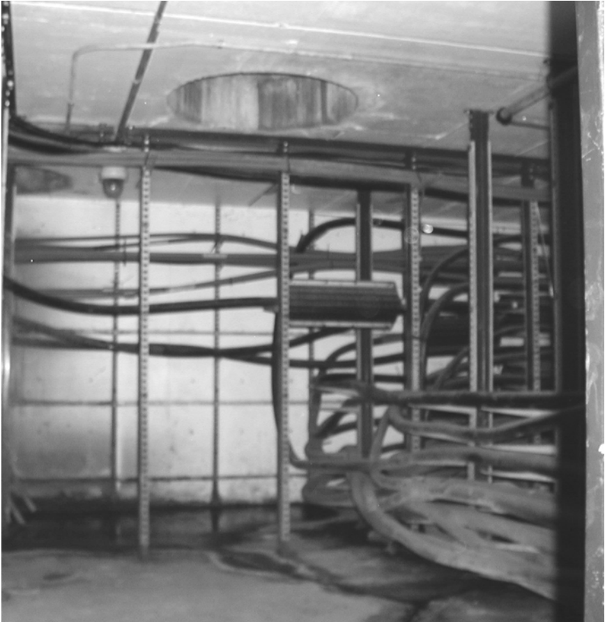
Figure C.7 Cable Vault (Inside View). Street Access is at Top
