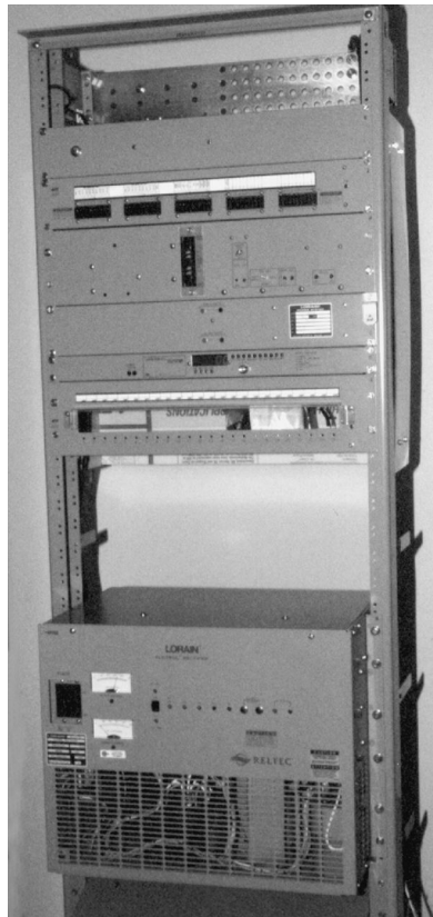
Figure R.4 Rectifiers
