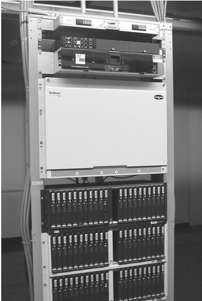
Figure D.31 DSLAM (Digital Subscriber Line-Access Multiplexer)
