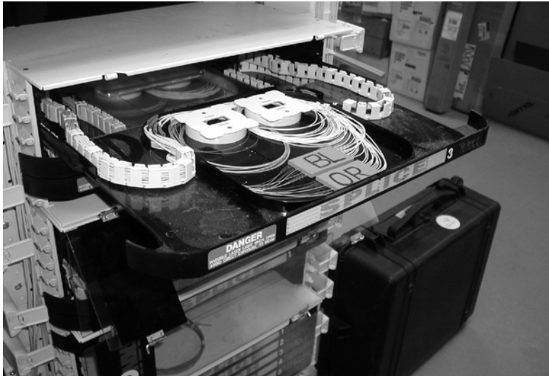
Figure S.19 Fiber-Optic Splice Tray
